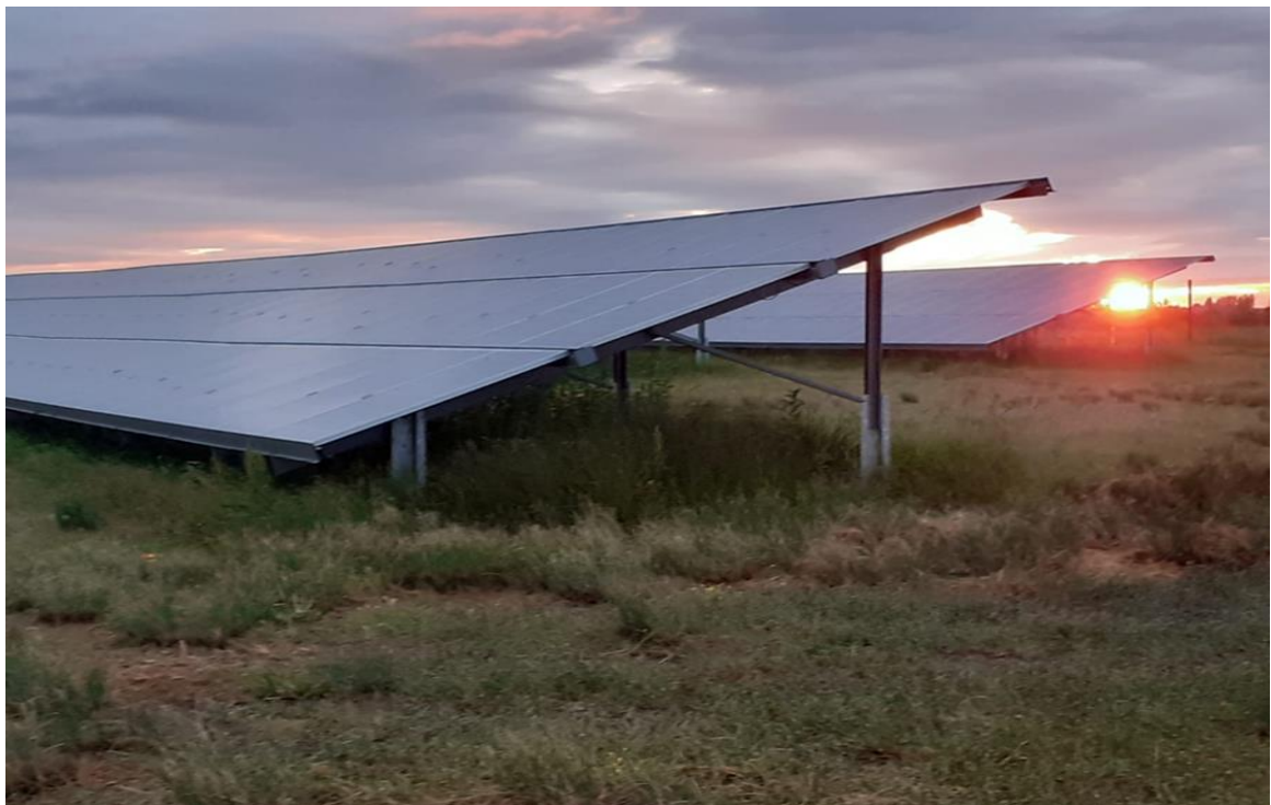
Photo Solar Farm at the former Gedling Colliery
